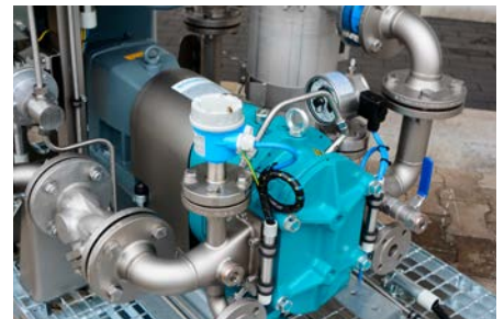
Pressure measurement by means of pressure transmitter
